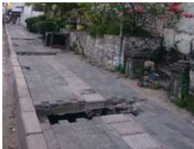
Figure 1. Condition of the pedestrian path in market area
