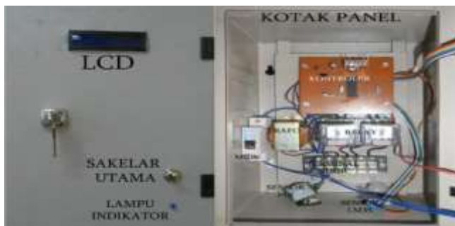
Figure 4 Overall Hardware View
