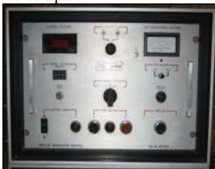
Figure 3. Front panel of the control console
