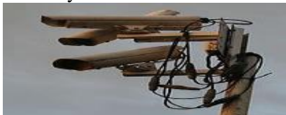
Fig. 1 Example of CCTV camera
