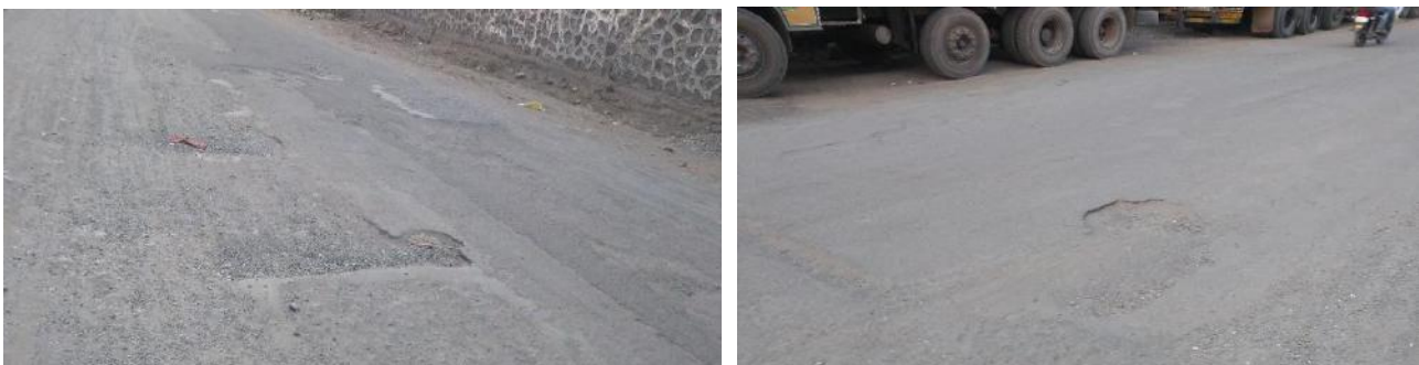
Figure 1. Potholes due to heavy transports & water logging.
