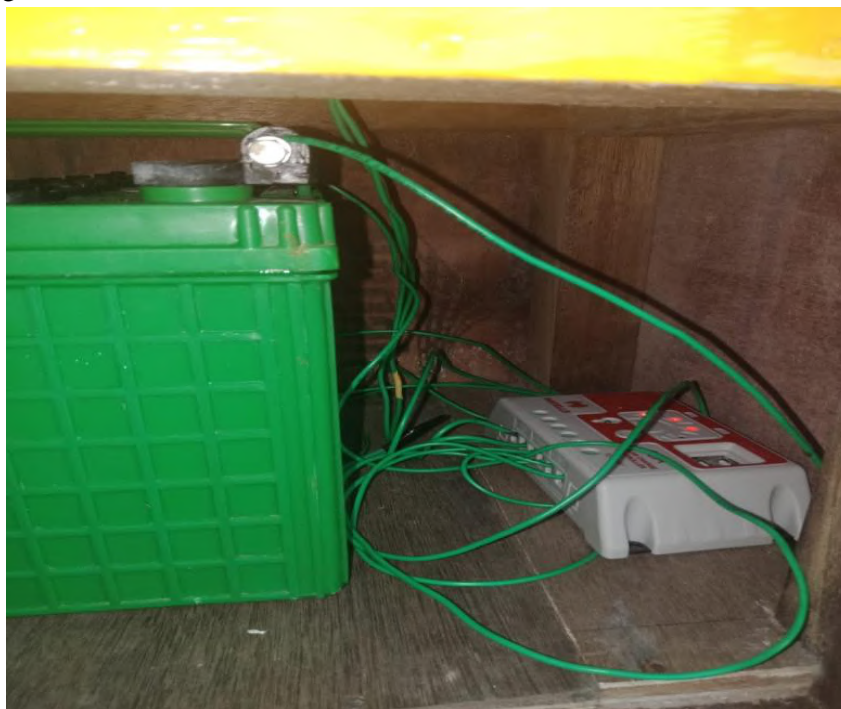
Figure 2. Solar charge controller with the battery and solar panel connections
