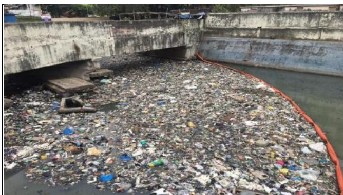
Fig. 6. Trash boom installed in drainage channel [35]
