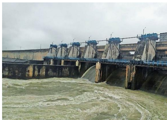
Figure 1. Downstream view of spillway gates of Chankapur Dam, Nashik District, Maharashtra, India
